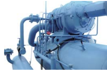
Original oil injection system
